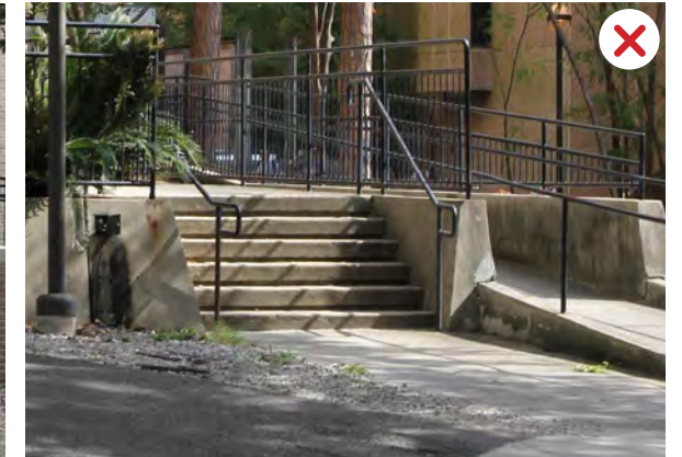
Building stairs with unnecessary railings and walls
