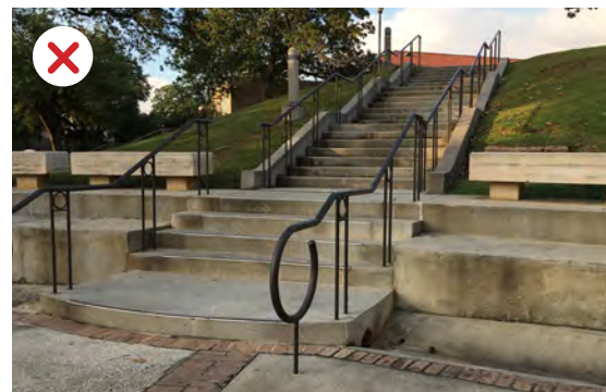
Stairs with unnecessary walls and ornamentation
