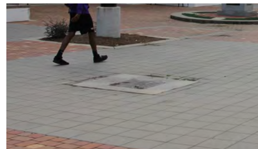
(Right) Avoid locating catch basins in paved areas. Where basins must be used, extend the paver surface to the basin rim to minimize disruption to the paving design.
