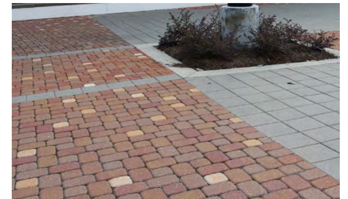
A variety of concrete paver types and colors in a plaza
