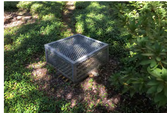
(Above left) Catch basins located in planted areas should have screen protection from plant litter.
